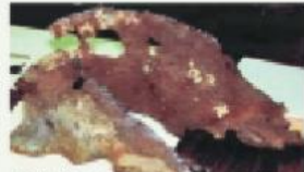
FEMA's May 2002 report documents evidence of severe high temperature corrosion attack on the steel.
